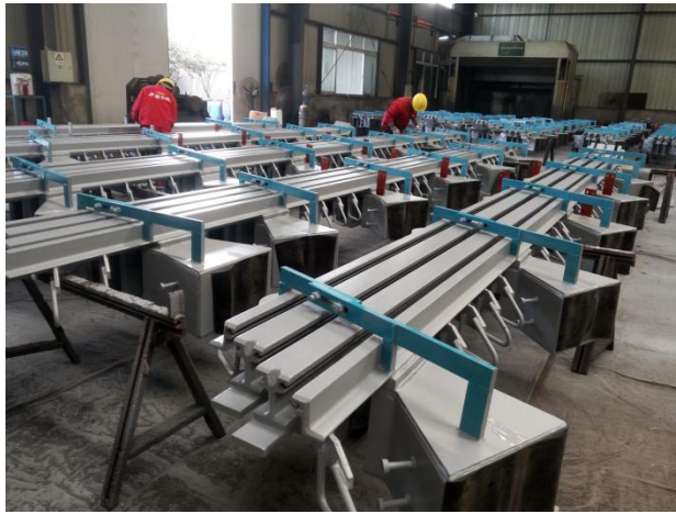
Painting of modular expansion joint at IEC workshop for NOH2 project in Doha Qatar, 2018
