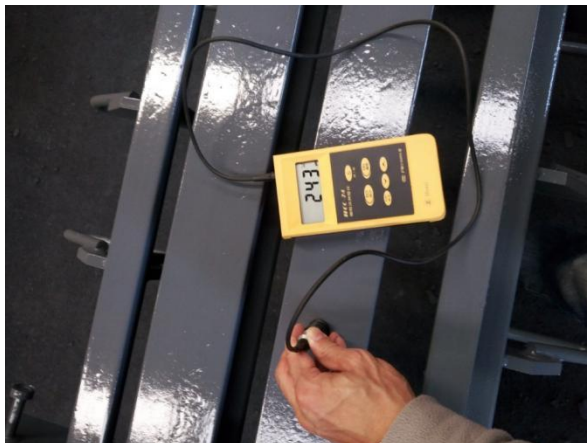
paint film thickness 243 microns (C5-MI) for E-ring road project in Doha Qatar, 2018
