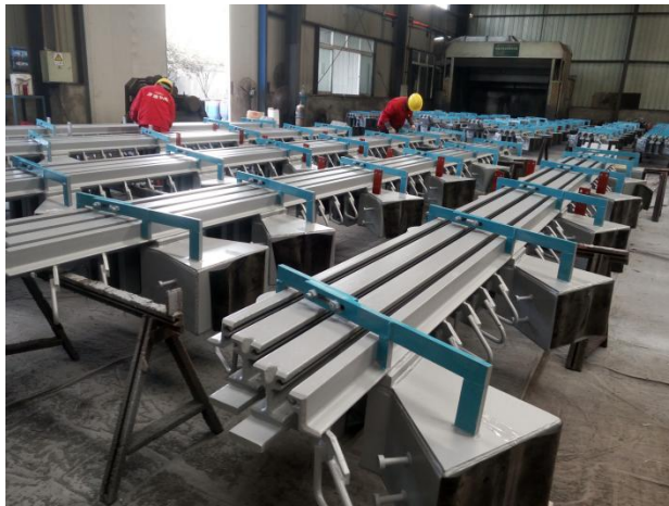
Painting of modular expansion joint at IEC workshop for NOH2 project in Doha Qatar, 2018
