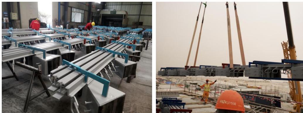
Over 550 meters of Swivel MBJS was supplied by IEC for NOH2 project, Qatar, 2017-2019
