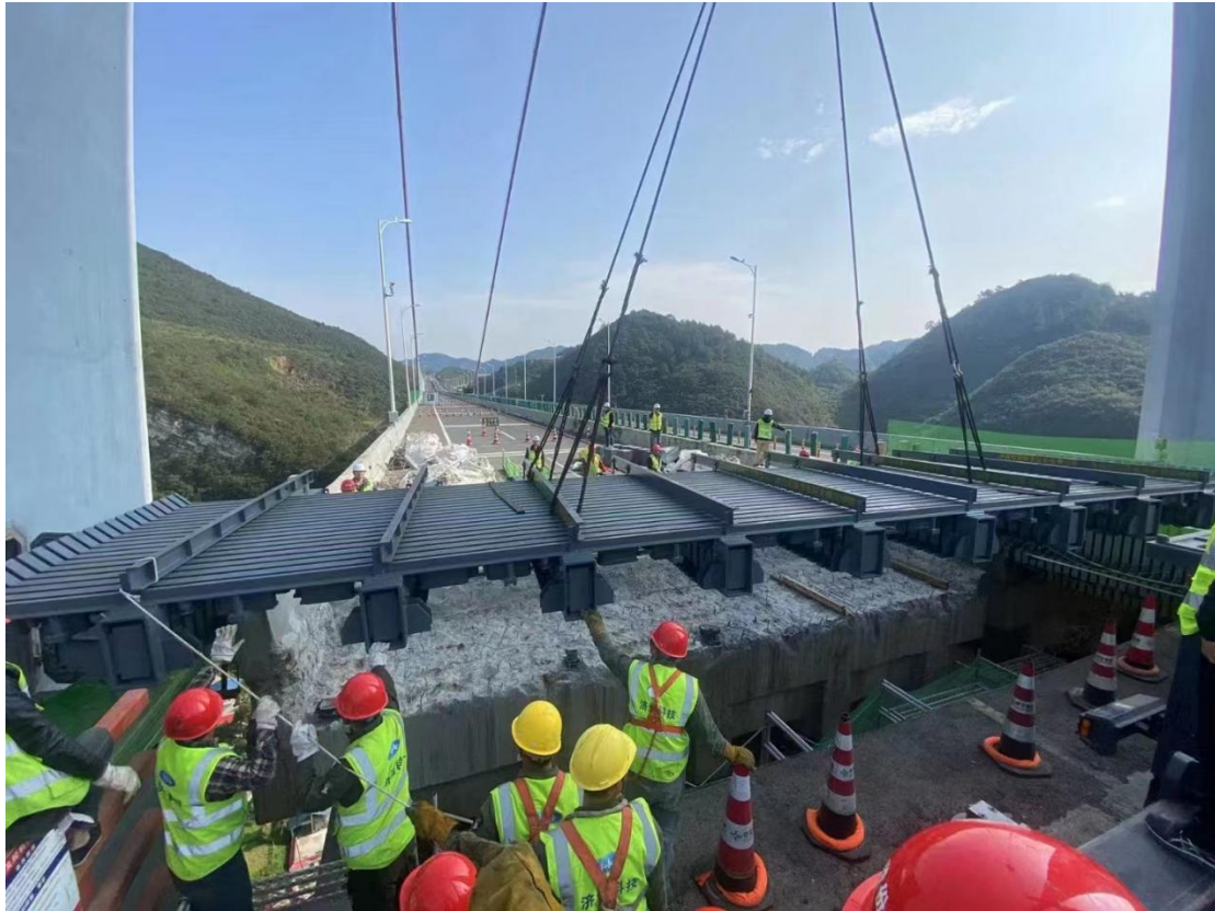
20-seal modular joint was lifted up for installation for Qingshui River Bridge, Guizhou Province, China
